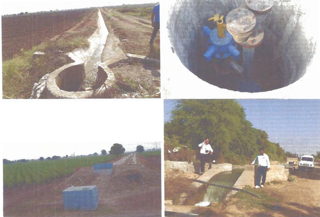
Pic 26. The Distribution System under Village Service Areas
