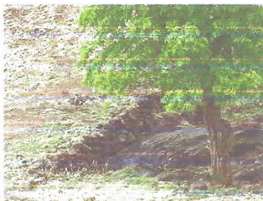
Pic 6. Catchment area treatment works in Rajasthan (Loose Boulder Structure, Water Harvesting Structure and Nala Bund)
