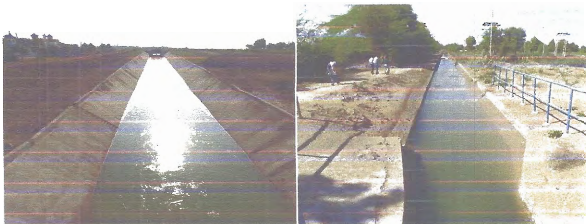
Pic 25. Water delivery network in Rajasthan
